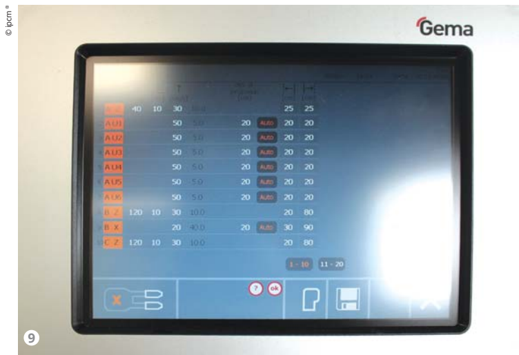
Figure 9: The control panel of the powder coating booth.
