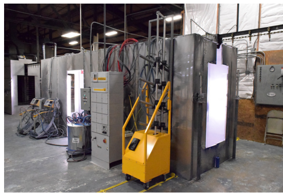
Figure 4 Matthews Industries had a Gema MultiStar automatic package that controls eight automatic powder spray guns mounted on a gun mover installed to increase product line density.
